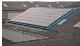
[太陽光発電10KWを設置]
